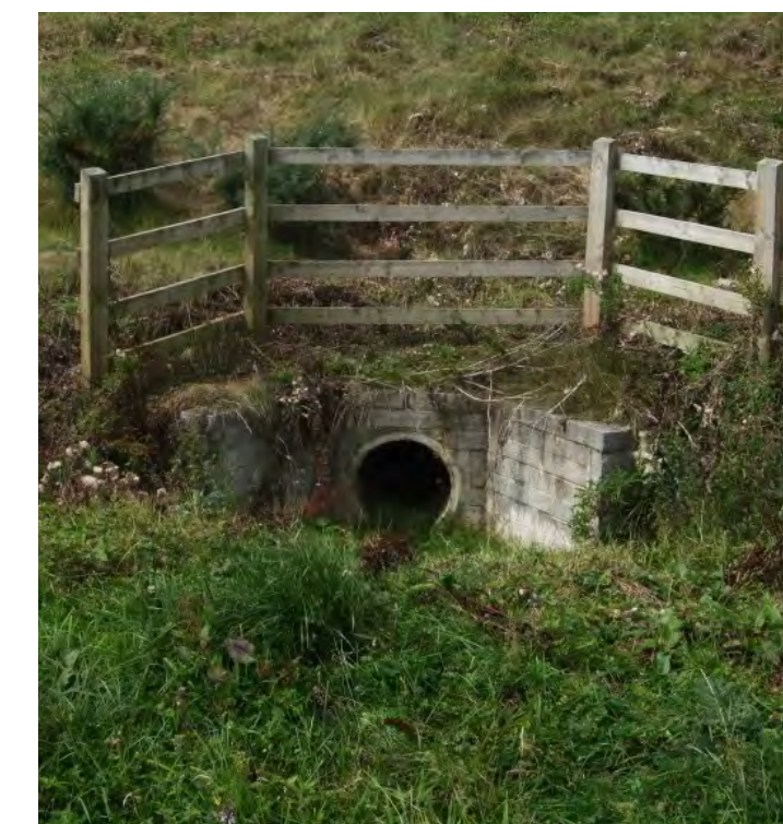
▲ Tunnels under roads help prevent badger deaths due to traffic
