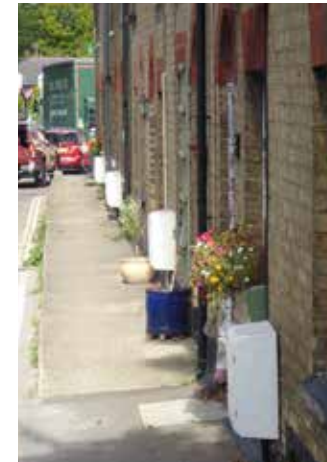
Figure 91: Meter boxes on Kingsland Terrace
