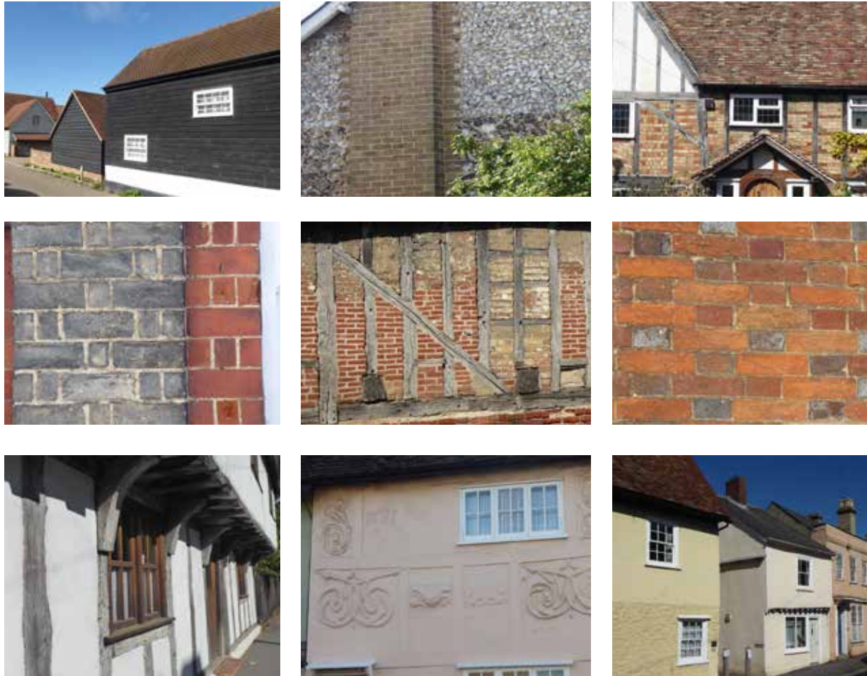
Figure 32: Examples of different wall materials within the Character Area . From left to right: Top Row Weatherboarding, flint and brick, timber Framing with sections of brick nogging and render infill. Middle Row, Rat Trap bond and grey brick, exposed timber with nogging, Flemish bond brickwork. Bottom row, exposed timber-framing with lime render, pargetting, rendered and jettiedhouse
